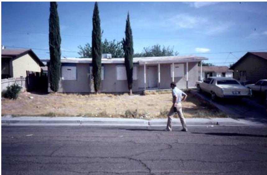
Figure 3-2 Differential settlement building damage
