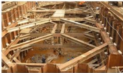
Some kinds of structure to prevent land slide.(for construction)
