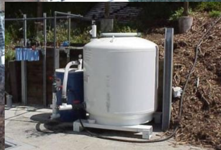
Treatment unit (GAC)
