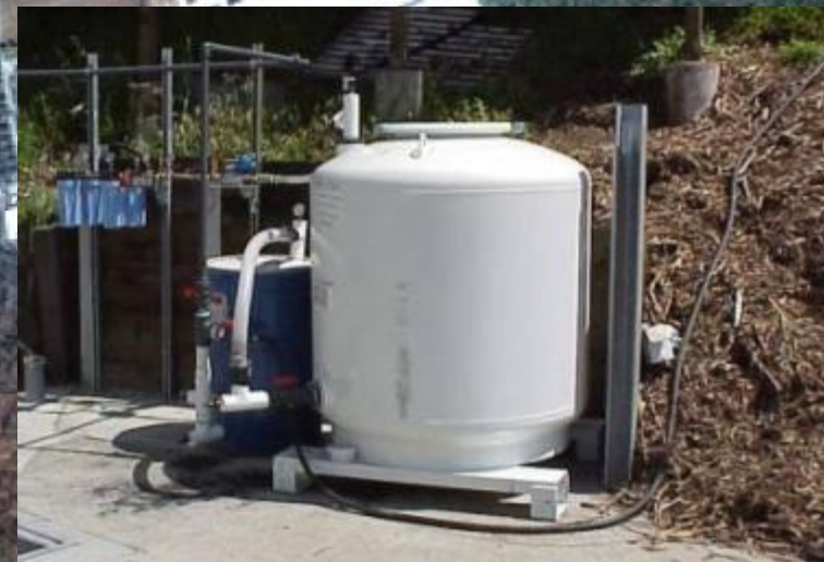
Treatment unit (GAC)
